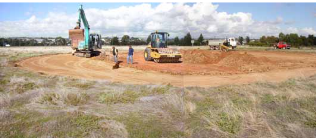
DTEI's team at work, under canine supervision, constructing the new vernal pool at Parafield Airport.
