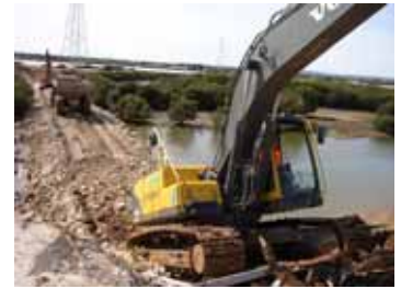
Starting to excavate the trench for the new pipe across Dry Creek
